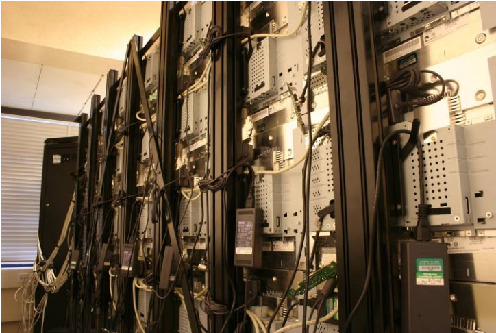
Figure 4 Rear view showing bracing
